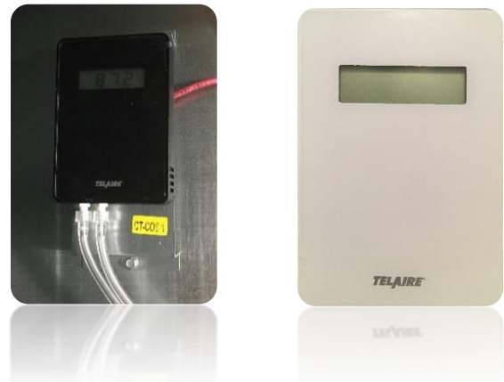
Figure 4. CO2 sensor located inside unit
