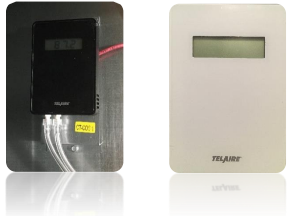
Figure 3. CO2 sensor located inside unit
