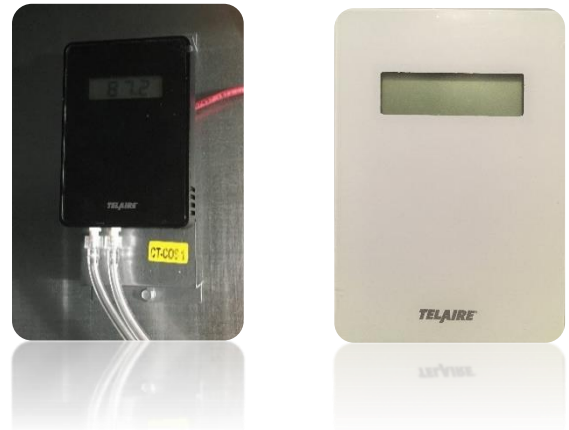
Figure 3. CO2 sensor located inside unit
