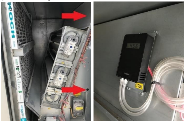
Figure 2. CO2 sensor location inside the unit
