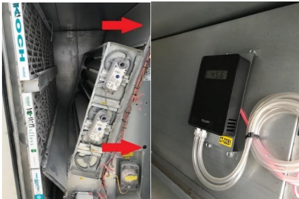
Figure 3. CO2 sensor location inside the unit
