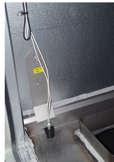
Figure 2. Float Switch Mounted and Control Wires Secured to Interior Cabinet Wall
