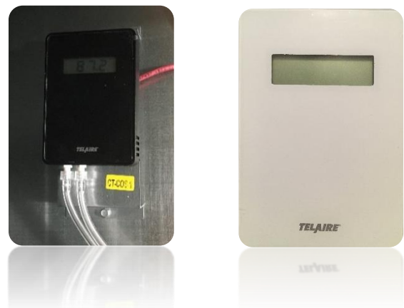
Figure 4. CO2 sensor located inside unit
