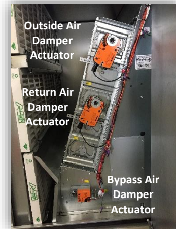
Figure 3. Damper Assembly and Actuators
