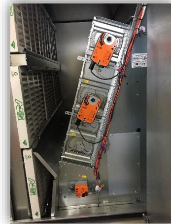
Figure 3. Damper Assembly and Actuators
