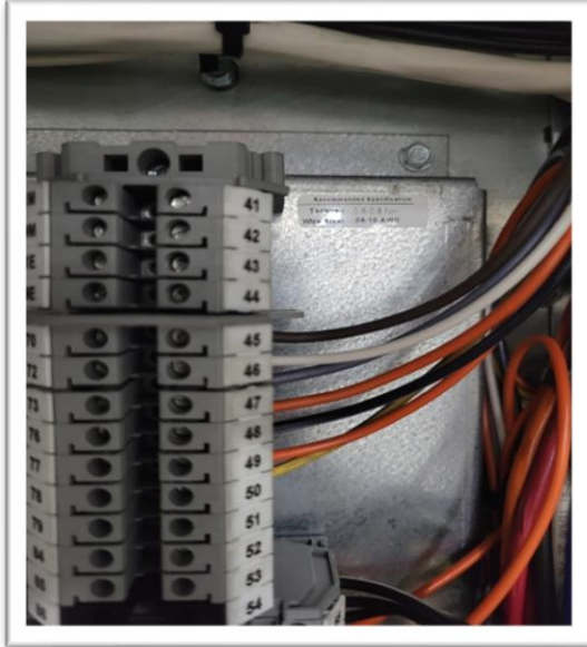
Figure 3. Sub-Panel Block Wiring
