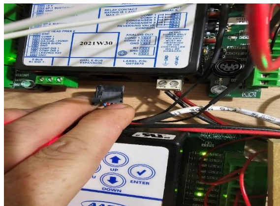
Figure 10: Ebus plug on bottom of VCCX/RSM modules
