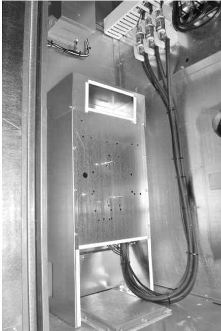
Figure 25 - Back View of Utility Entry and Power Switch from Control Compartment ( 70-140 ton Units)
