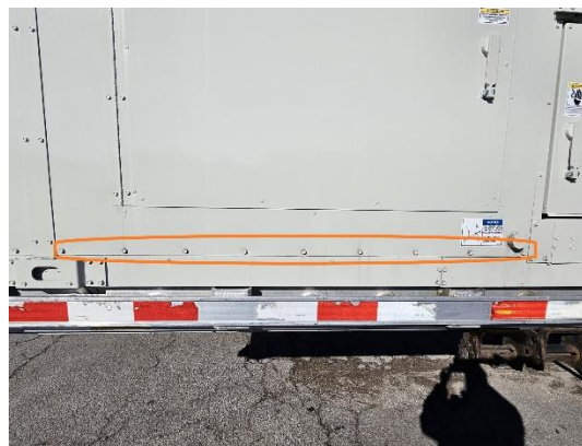
Fig. 6. Screw Removal Coil Cabinet Bottom Panel
