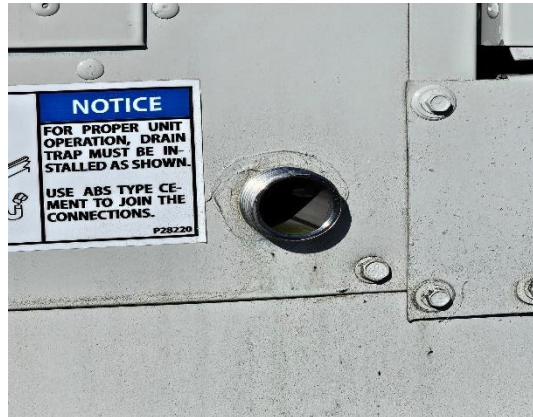
Fig. 9. Drain Spout Caulking Removal
